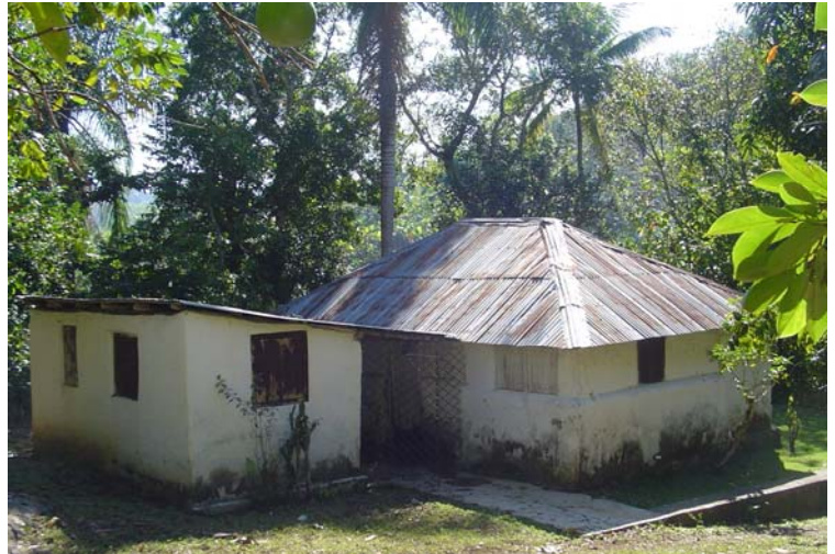
Small house on FFH land to be used as a temporary clinic during construction.
