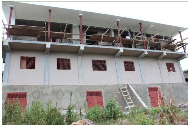
Iron posts installed along the sides of the back porch of the residence. Horizontal railings will be attached to the posts for safety.
