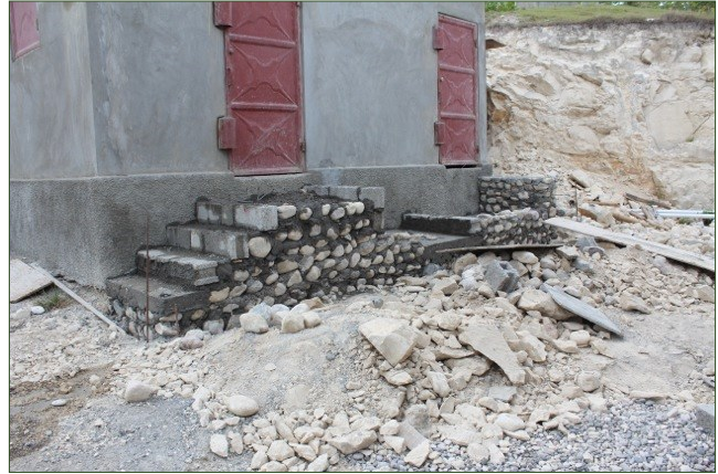
Partially completed steps leading up to the doors of the storage depot. The electrical system is in the room on the left and the water filters are in the room on the right.
