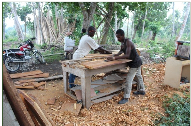
Carpenters working with hand tools to prepare wood for the windows of the clinic
